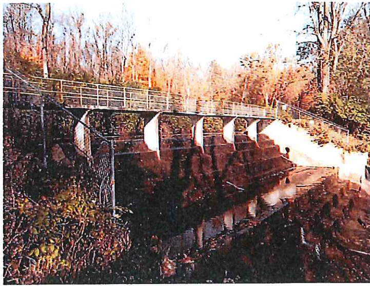
8. Spillway located on the canal. This is the only outlet for Echo Lake and Franz Pond.
