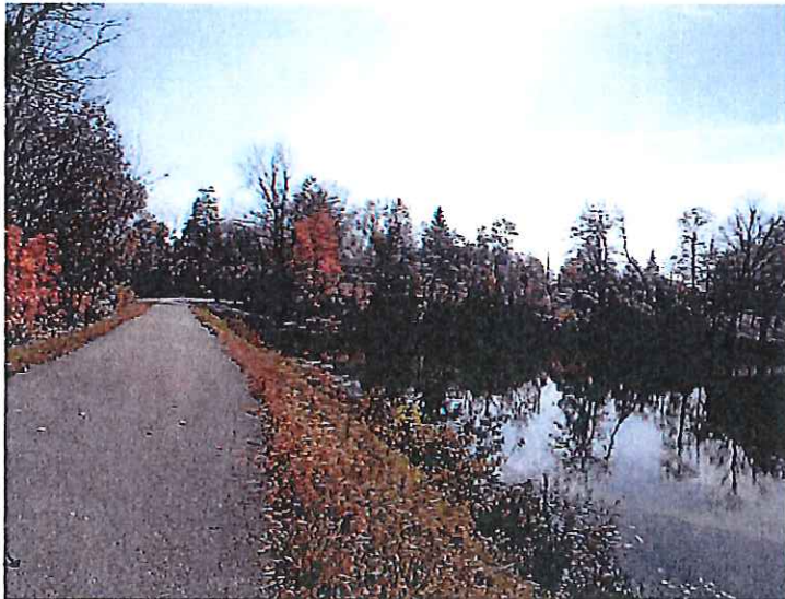
2. Crest and upstream slope looking towards the right end of the dam. Note the brush on the upstream slope.
