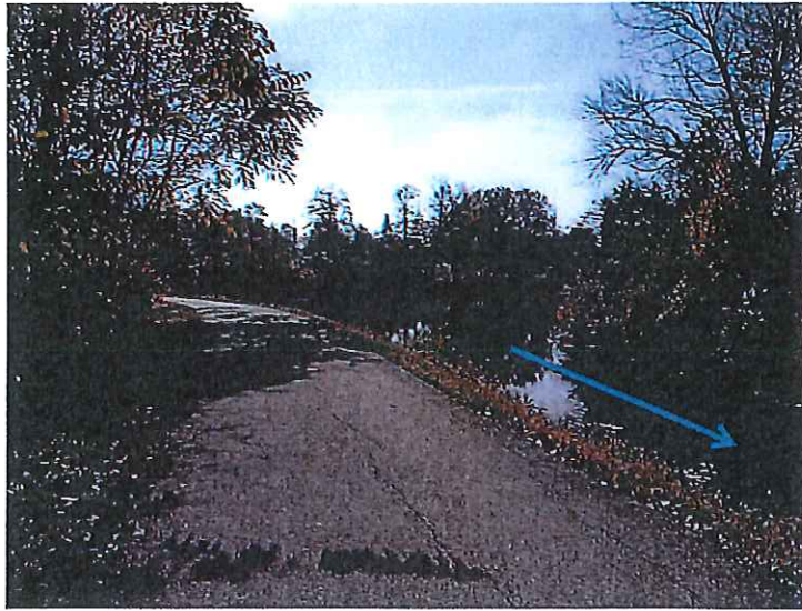
1. Crest looking towards the right end of the dam. Also note the inlet of the canal to Echo Lake.
