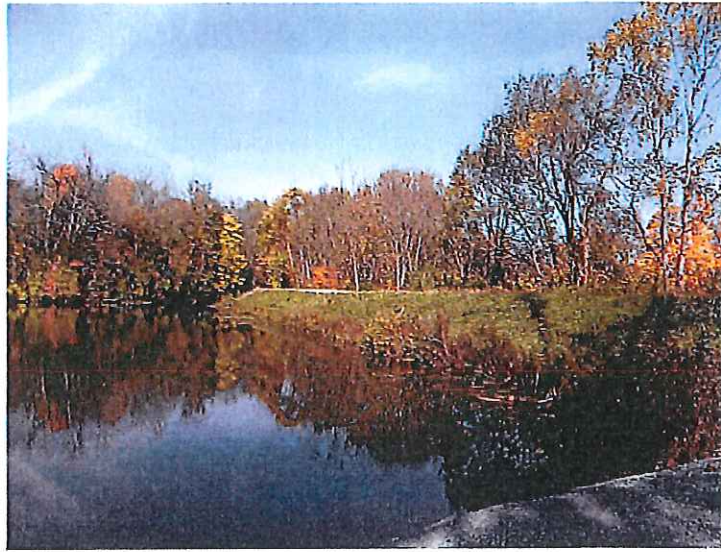
4. Upstream slope as viewed from the boat ramp at the right end of the dam. Note the brush along the shoreline.
