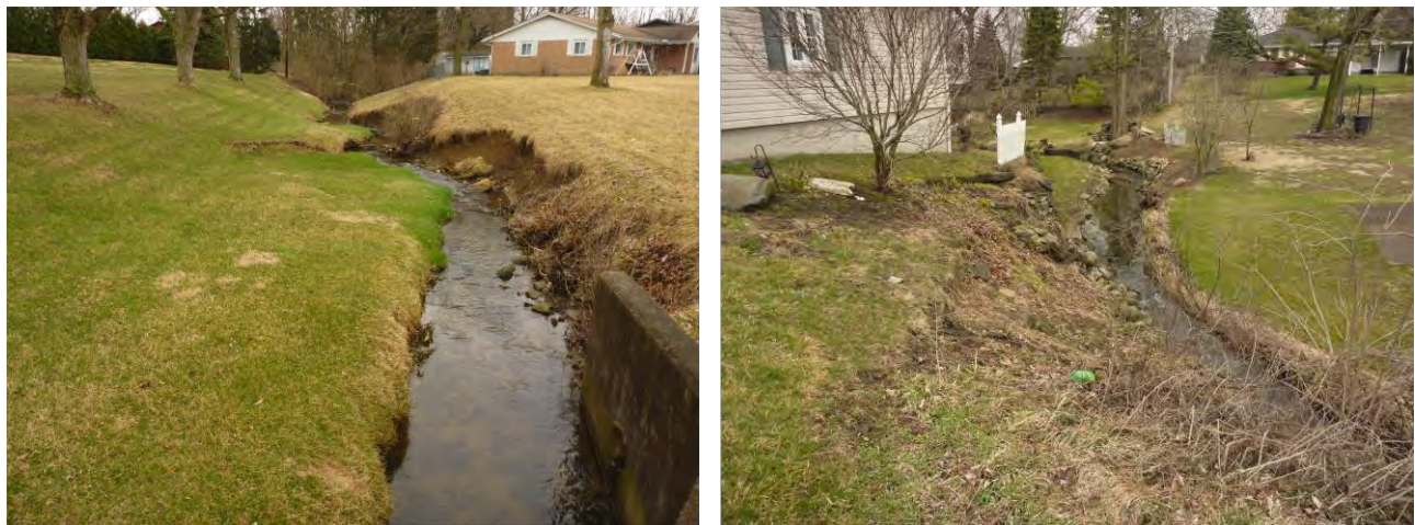
Figure 8 Significant Bank Erosion Along Peters Street Ditch to the South
