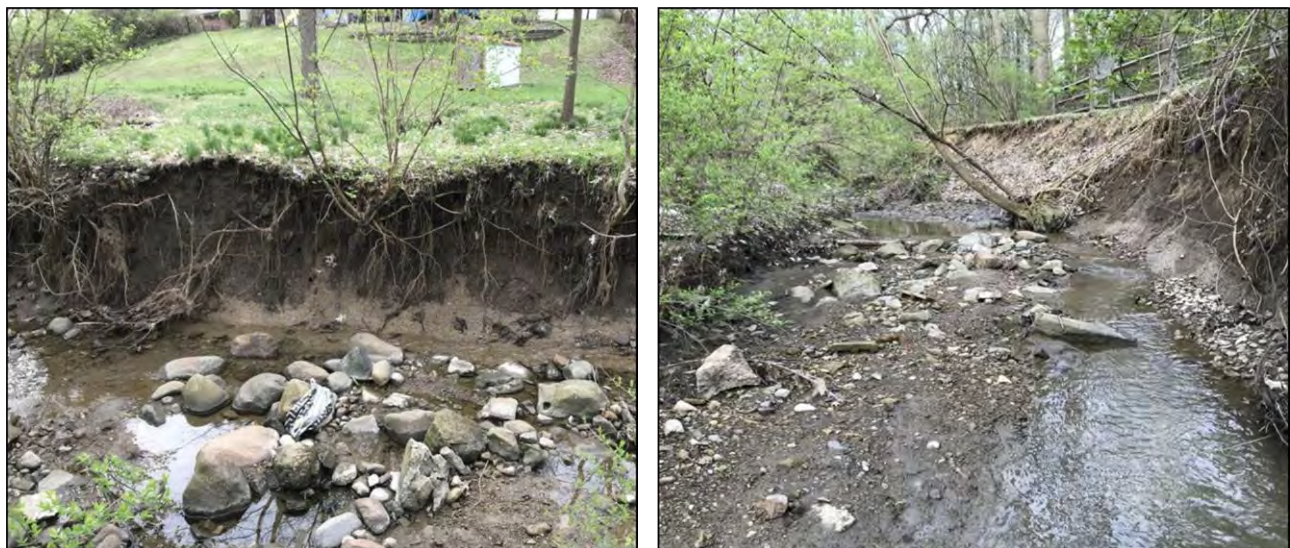
Figure 4 Significant Bank Erosion Along Franz Pond Ditch
